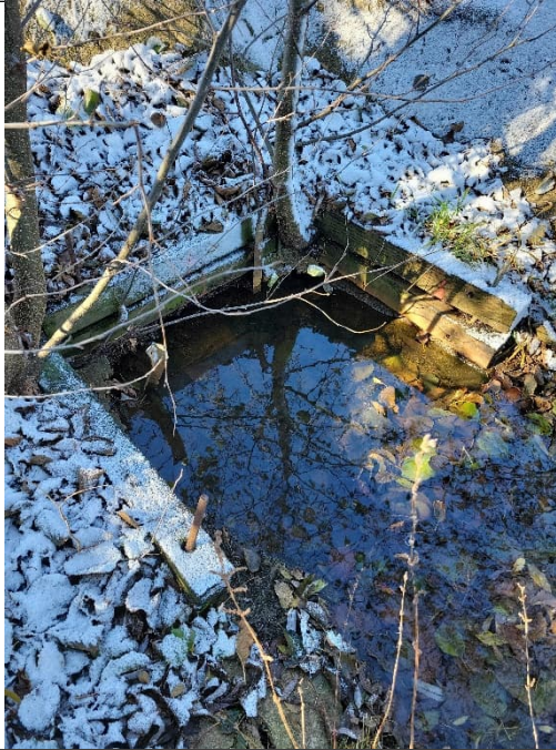
Photo 9: Outlet end of hydraulic outlet. No observable flow. Crown of pipe visible, submerged under lake water level. Debris buildup visible under water in channel from pipe to lake.
