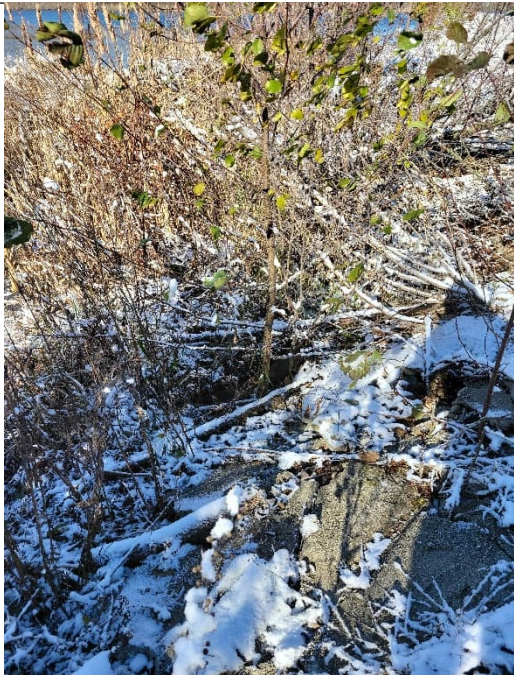
Photo 7: Inlet end of hydraulic outlet looking NW. Buildup of vegetative debris around trash guard/riser structure and deteriorating concrete along slope between structure and perimeter road.
