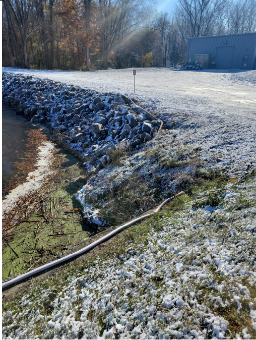
Photo 1: Soil covering riprap on outboard slope in NW corner.
