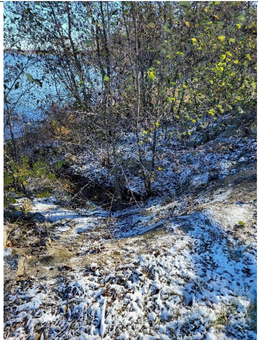
Photo 8: Outlet end of hydraulic outlet looking E towards Morrow Lake from perimeter road. Riprap and concrete protection in fair condition.
