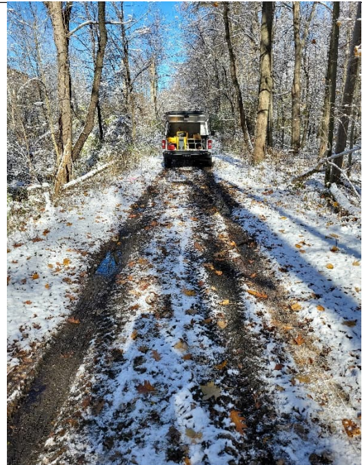
Photo 12: Road along western perimeter looking N. Vehicular rutting visible.
